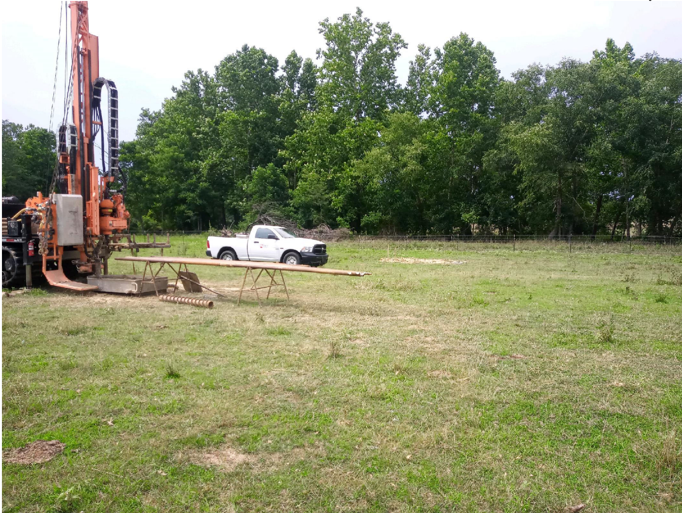
Location of borings 1, 2, and 3. South end of proposed new bridge location looking north. (July 2023).
