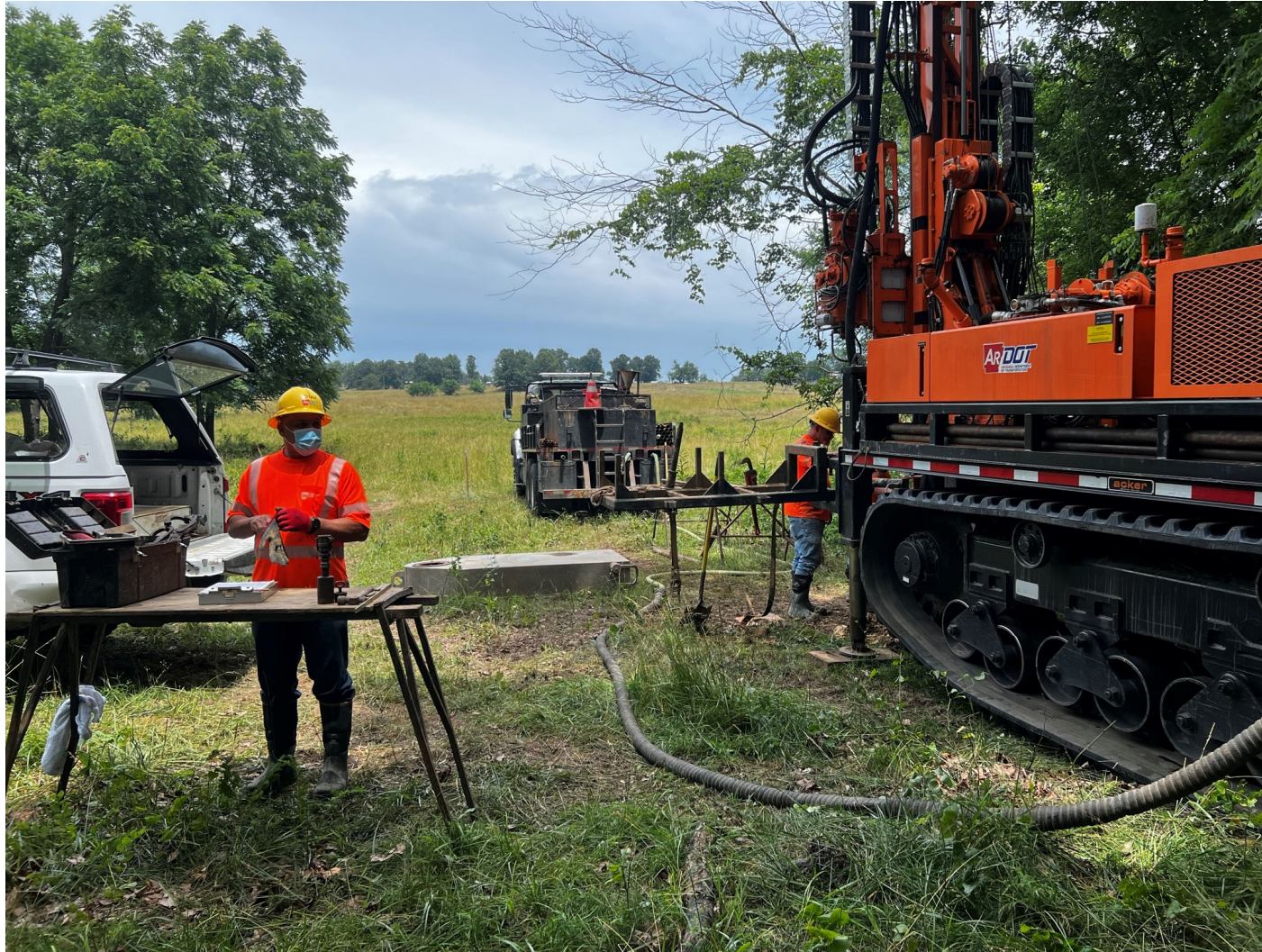
Looking north from north bank towards proposed location for the north bridge end (June 2023).
