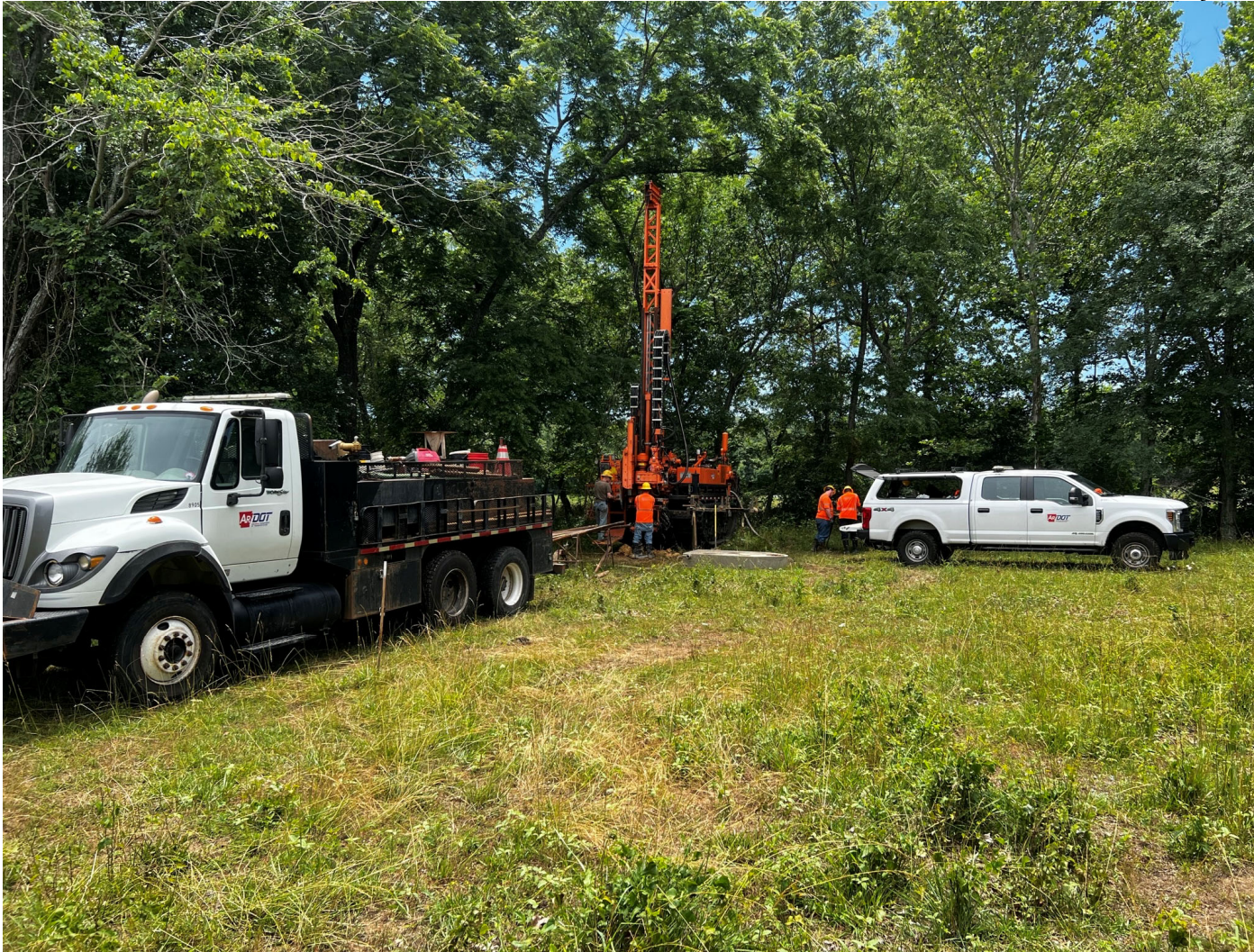
Location of borings 4 and 5. North end of proposed new bridge location looking south. (June 2023).
