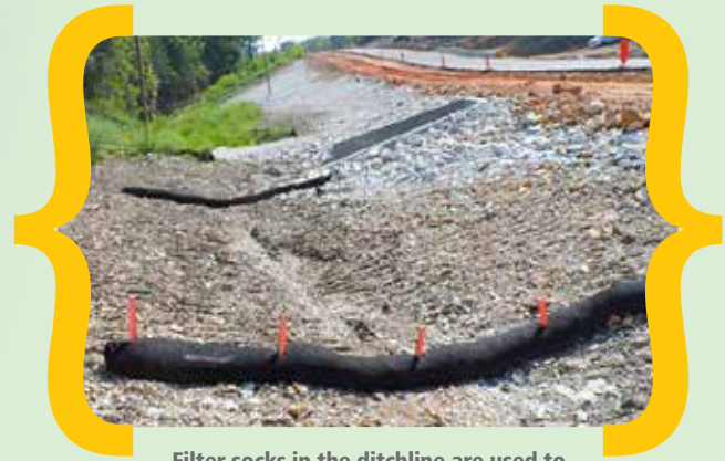
Filter socks in the ditchline are used to capture and treat stormwater runoff.
