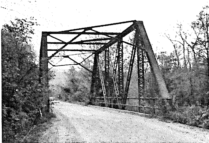
Bridge No. 15748, Type 310, steel through truss, Pratt through truss. Perry County Road 64 over Cypress Creek. Note skewed construction.
