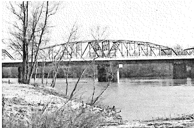
Bridge 483, Type 310, steel through truss, turn span. U.S. Highway 67 over Black River, Pocahontas, Randolph County. Added one-way lane this side of old bridge. Note turn mechanism pier, center of main span.
