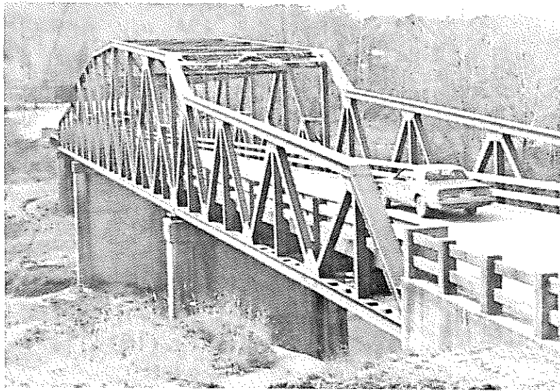
Bridge No. 1689, Type 310, steel through truss, Pennsylvania truss. State Highway 7 over Buffalo River, Newton County.
