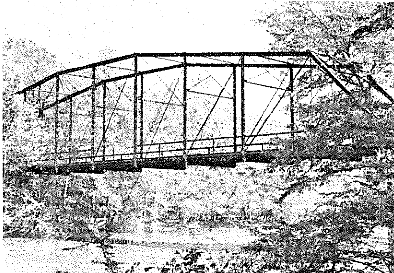
Bridge No. 20103, Type 310, steel through truss, Camelback truss. Clark County Road 479 over Little Missouri River.
