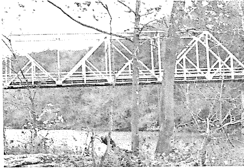
Bridge No. 1597, Type 310, steel through truss, Baltimore truss. State Highway 123 over Big Piney Creek, Johnson County.
