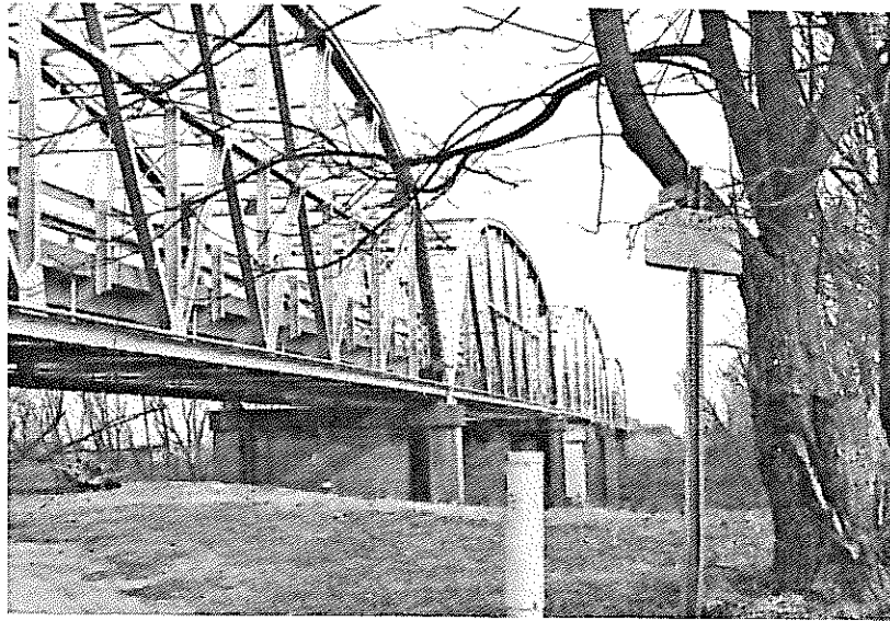
Bridge No. 1391, Type 310, steel through truss, Parker truss, turn span. U.S. Highway 70 over St. Francis River, St. Francis County.
