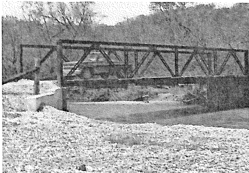
Bridge No. 10604, Type 310, steel Pony truss, Bedley truss. Benton County Road 29 over Spavina Creek.
