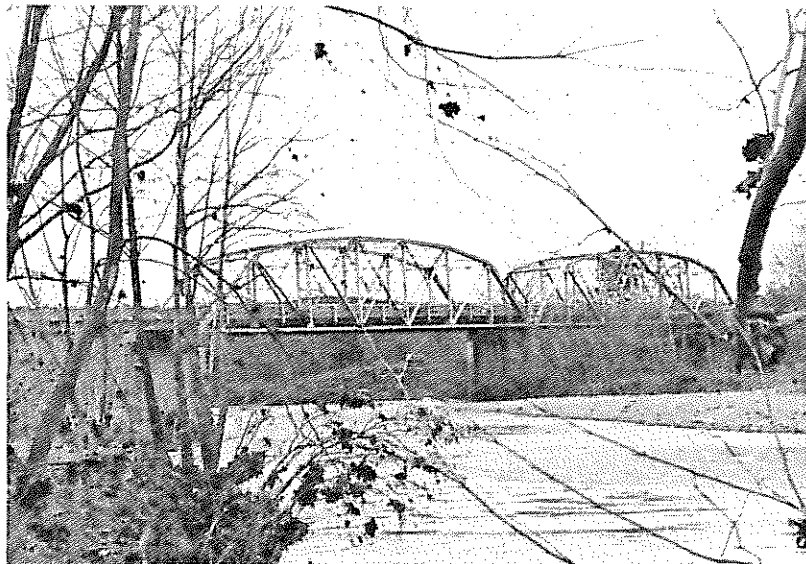
Bridge No. 1811, Type 310, steel through truss, Pennsylvania truss. State Highway 59 over Lee Creek, Crawford County.
