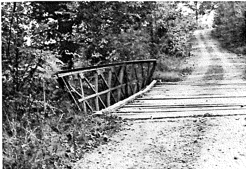
Bridge No. 17743, Type 310, steel Pony truss, double-intersection Warren truss. Yell County Road 222 over Achmun Creek.
