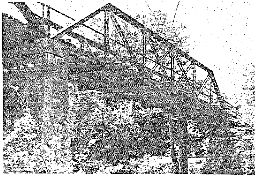
Bridge No. 16149, Type 310, steel Pony truss, Pratt truss. Polk County Road 38 over Mountain Fork of Little River.
