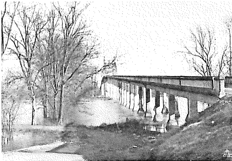
Bridge No. 613, Type 310, steel through truss, double arch cantilever main span. U.S. Highway 64, over White River, Augusta, Woodruff County.
