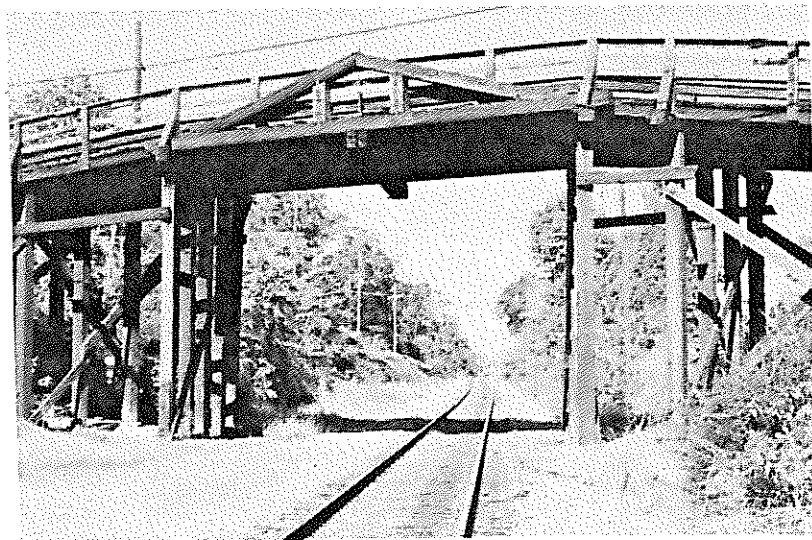
Bridge No. 19417, Type 710, timber truss, modified King-post truss. W. 14th. St. over MoPac R.R. North Little Rock, Pulaski County.
