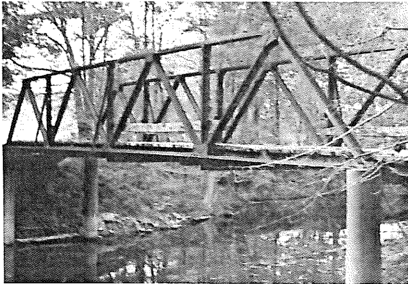
Bridge No. 16902, Type 310, steel pony truss, Warren truss. Sevier County Road 139 over Little Cossatot River.
