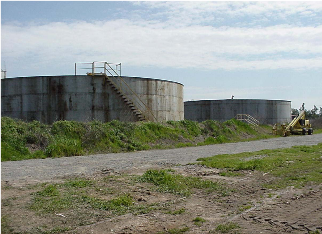
Liquid storage tanks located near the main warehouse
