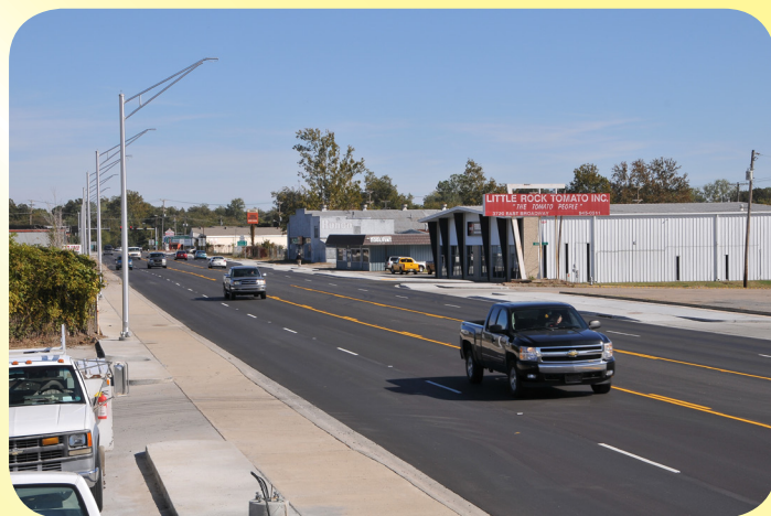
Two phases of work included $12.4 million to widen Highway 70 to five lanes from Interstate 30 eastward to Highway 165. Over 20,000 vehicles travel the heavily commercialized roadway on a daily basis.
