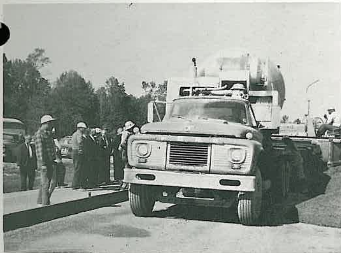
A central mix plant. Trucks are used to haul the mix to the construction site.
