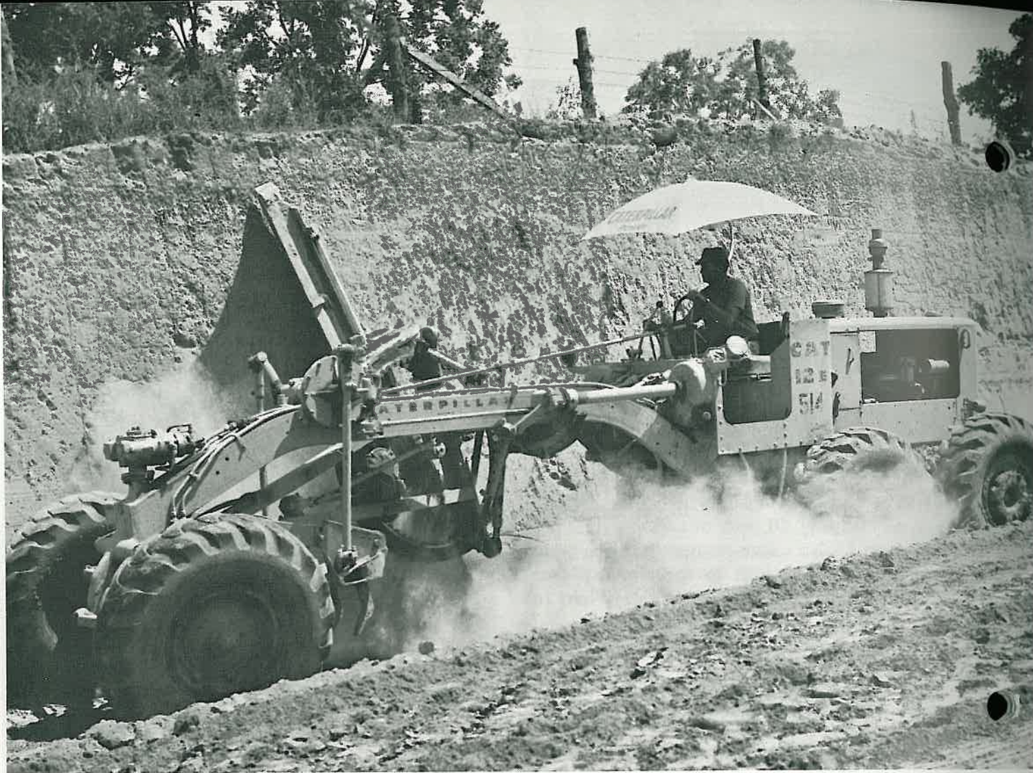
A straight cut is made to avoid erosion of the hillside on Highway 334.
