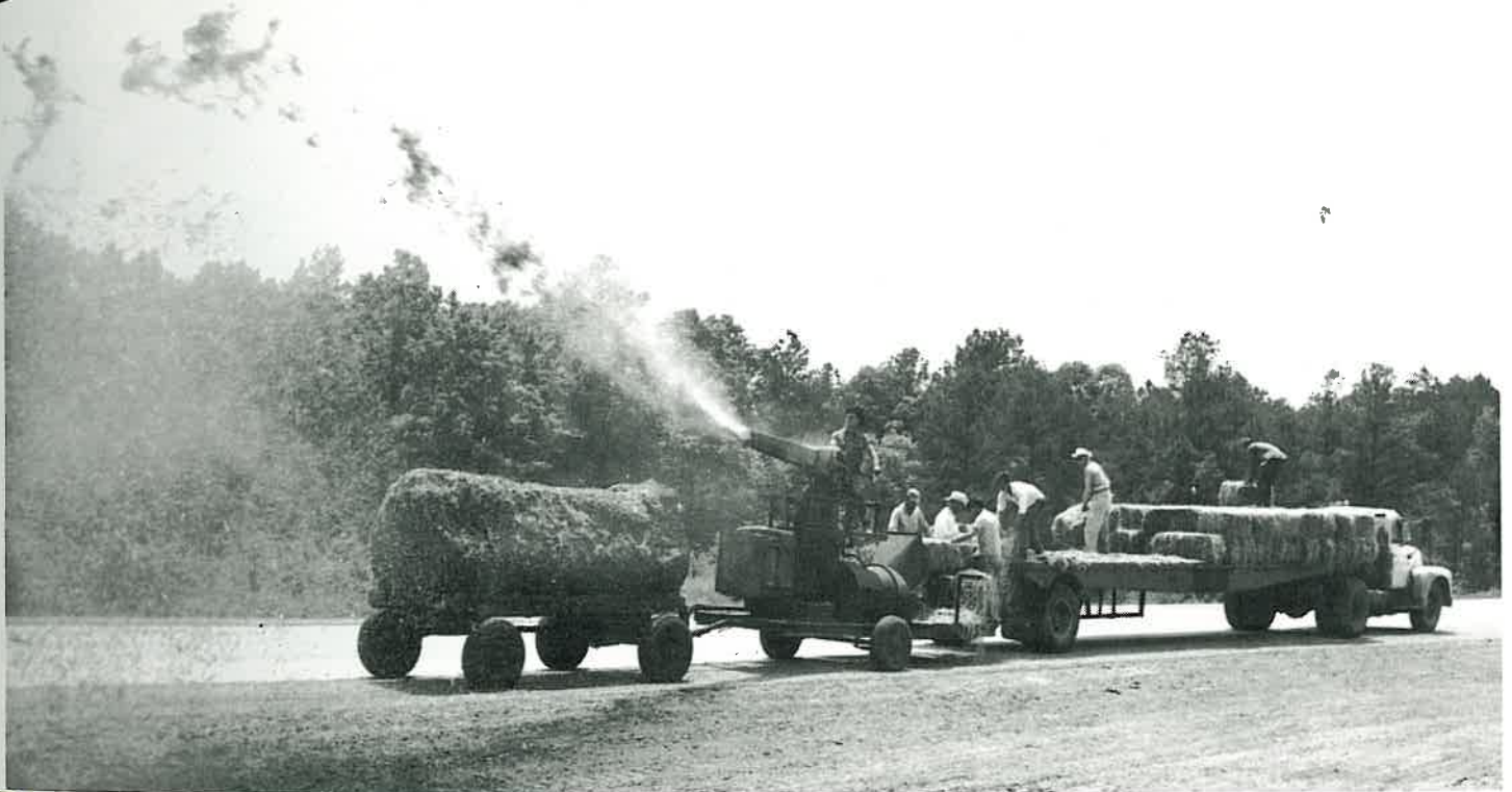
you happen to be working downwind of this seeding machine, you can be tarred and strawed in no time. A mixture of grass seeds, straw and asphalt are sprayed on shoulders of interstate project between Fulton and Texarkana. The straw and asphalt seal and hold seeds until they take root.
