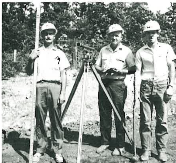
C. A. Ward, Imboden; J. E. Pickett, Black Rock; and J. R. Foley, Imboden set finished grade on a construction project on Highway 93 from Dalton to the Missouri line in Randolph County.
