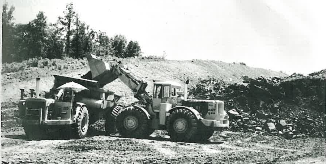
Construction scene from the relocation of U.S. 67 from the Pulaski-Lonoke County line to the junction with U.S. 64 west of Beebe. Work in progress above is between Jacksonville and Cabot. Glenn Cotham is the resident engineer.
