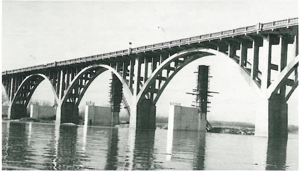
Piers for the new Garrison Avenue (U.S. 64) bridge rise in the air under and immediately beside the present bridge.
