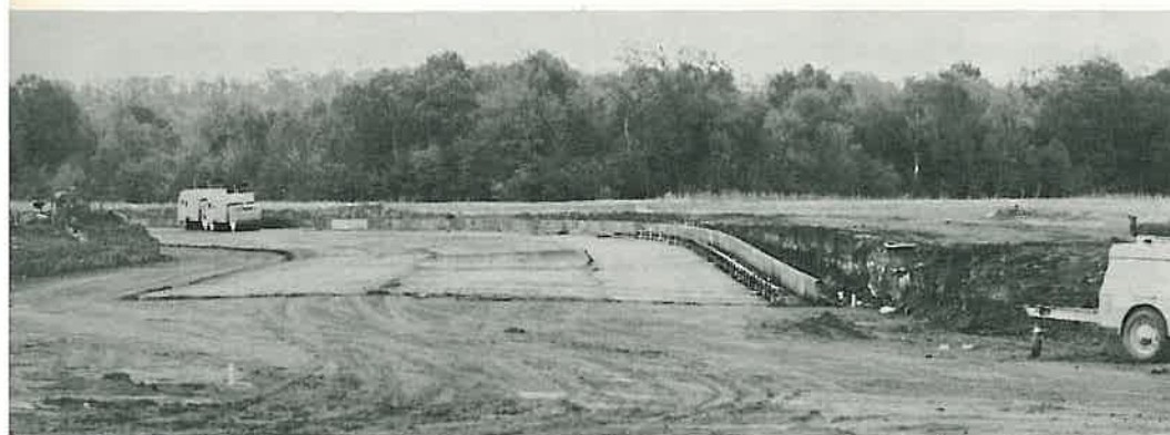
Putting down the base course on Highway 7 near the junction of Highway 124 on the campus of Arkansas Tech.
