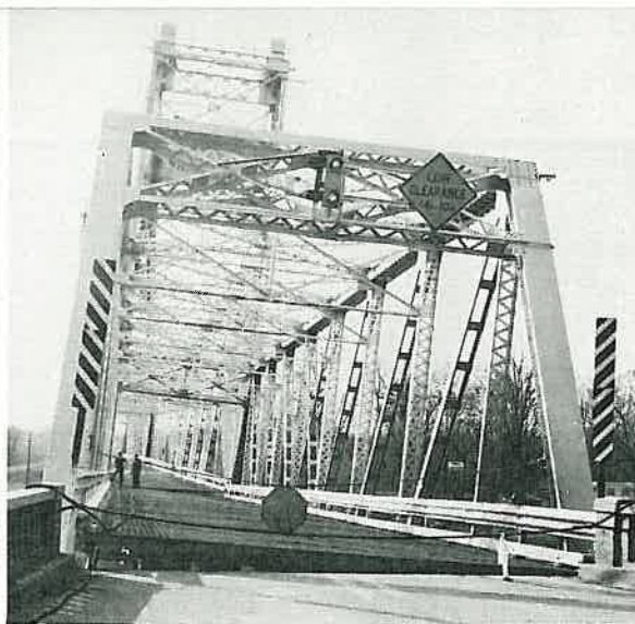
The east tower of the drawbridge lists to the north after pier settled.
