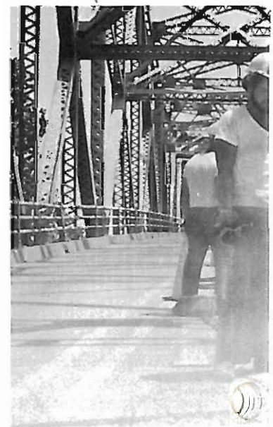
Bridge crews continued with scheduled maintenance, but were being called out to handle emergency repairs.
