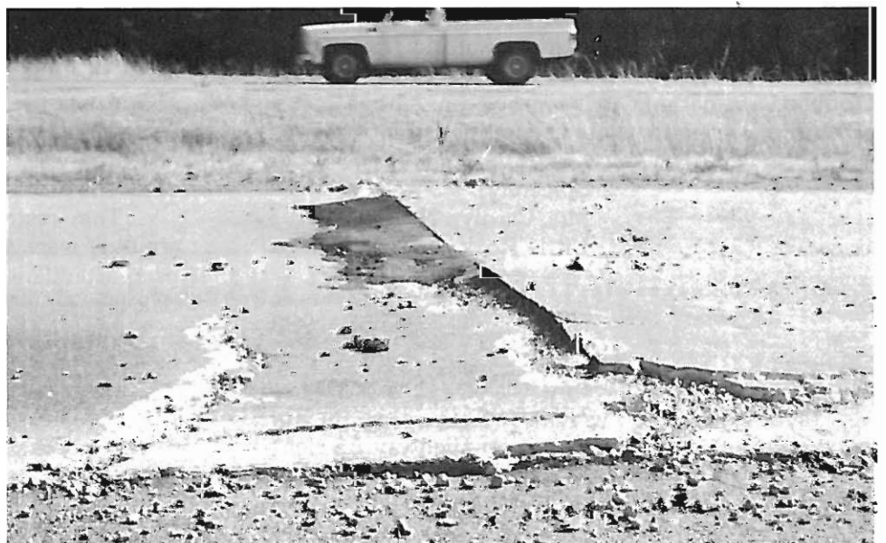
Pavement blow-ups, like this one on Interstate 40 near Morgan, became a common sight for motorists during the record heat wave.
