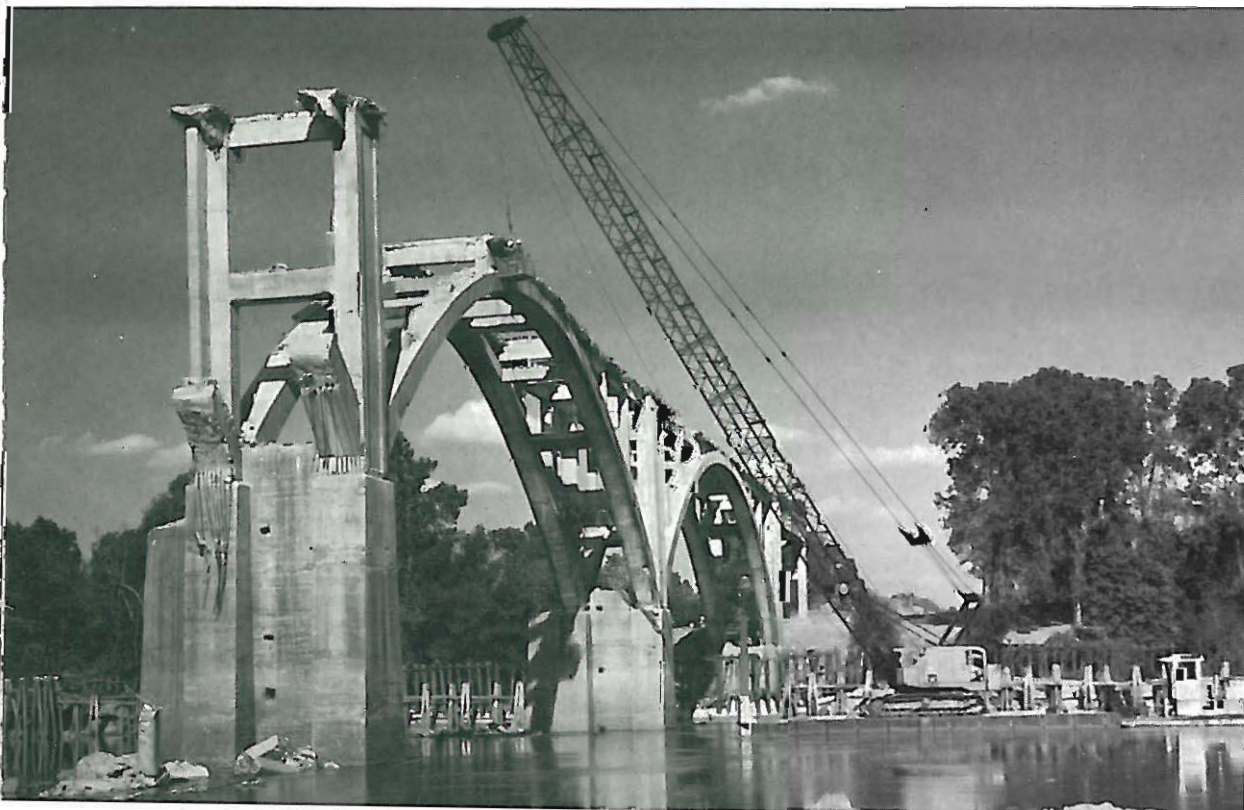
U.S. 67 Red River Bridge near Fulton being demolished after one of the main piers sank several feet. This bridge was constructed in 1929. The new bridge to be constructed will cost $3.5 million.
