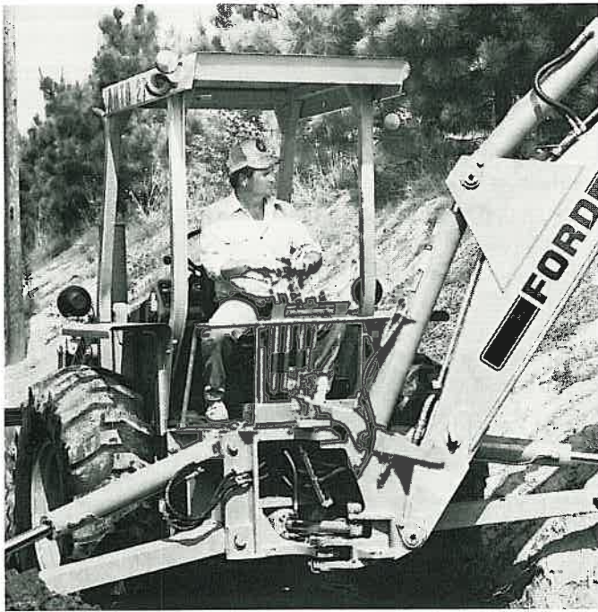
Backhoe Operator Charles Harvill of the Greene County Area Crew uses his Fridays off to get personal business taken care of.
