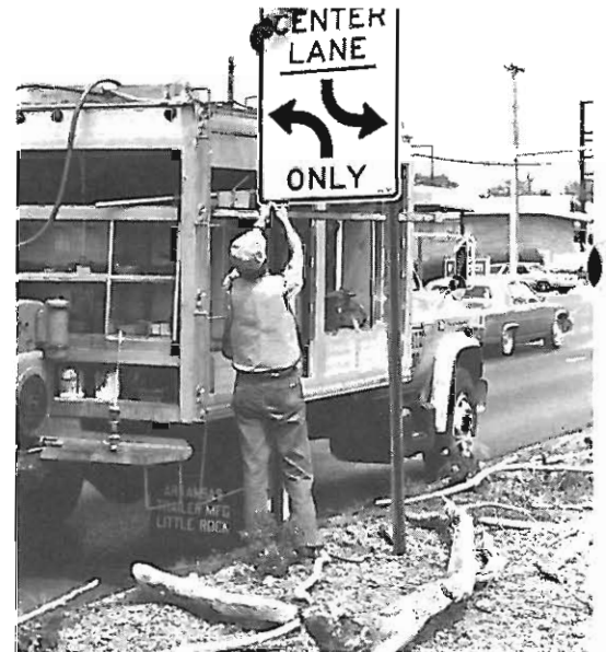
C.E. Pectol, top, signman with 31 years of service, and J.R. Smith, dozer operator, erect signs along downtown site in Batesville.
