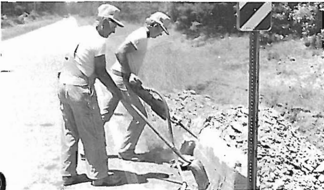
Charles Riley, left, 7 years service, and Kerry Blair, 10 years service, both Rough Carpenters, tear out concrete headwall on Highway 28.
