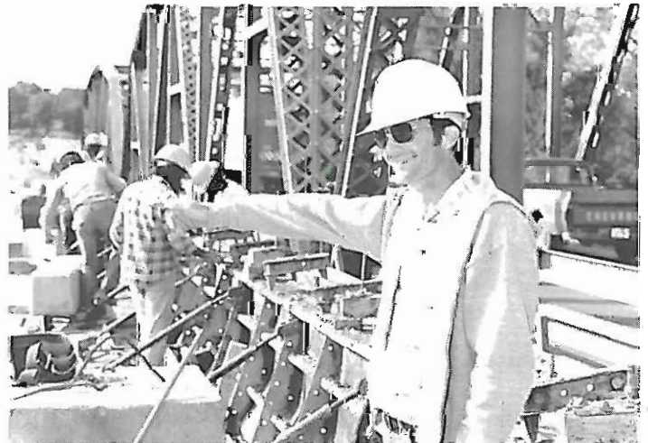
Walter Hamm, senior construction aide with 7 years, oversees work on the Highway 67 bridge at Pocahontas.
