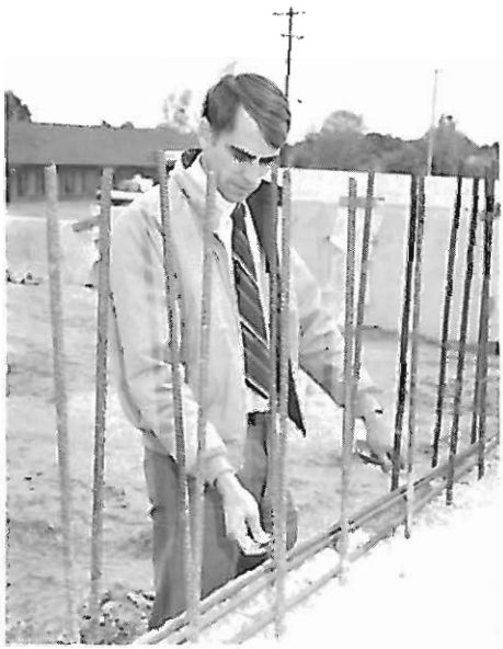
Joe Barnett, District Engineer with 15 years service, checks spacing on reinforcing steel.
