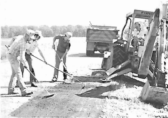
(L-R) David Cooper, truck dr.; Byron Hanson, general laborer; Jerry Easley, motor patrol operator; and Jim Dooley, backhoe operator, repair highway.
