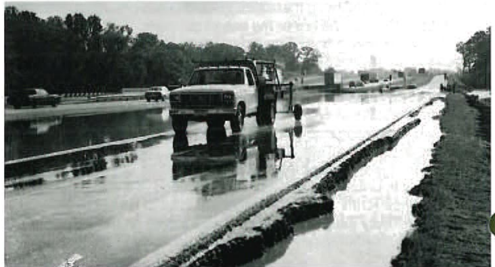
Shoulders along the highways were completely washed away following flash floods.
