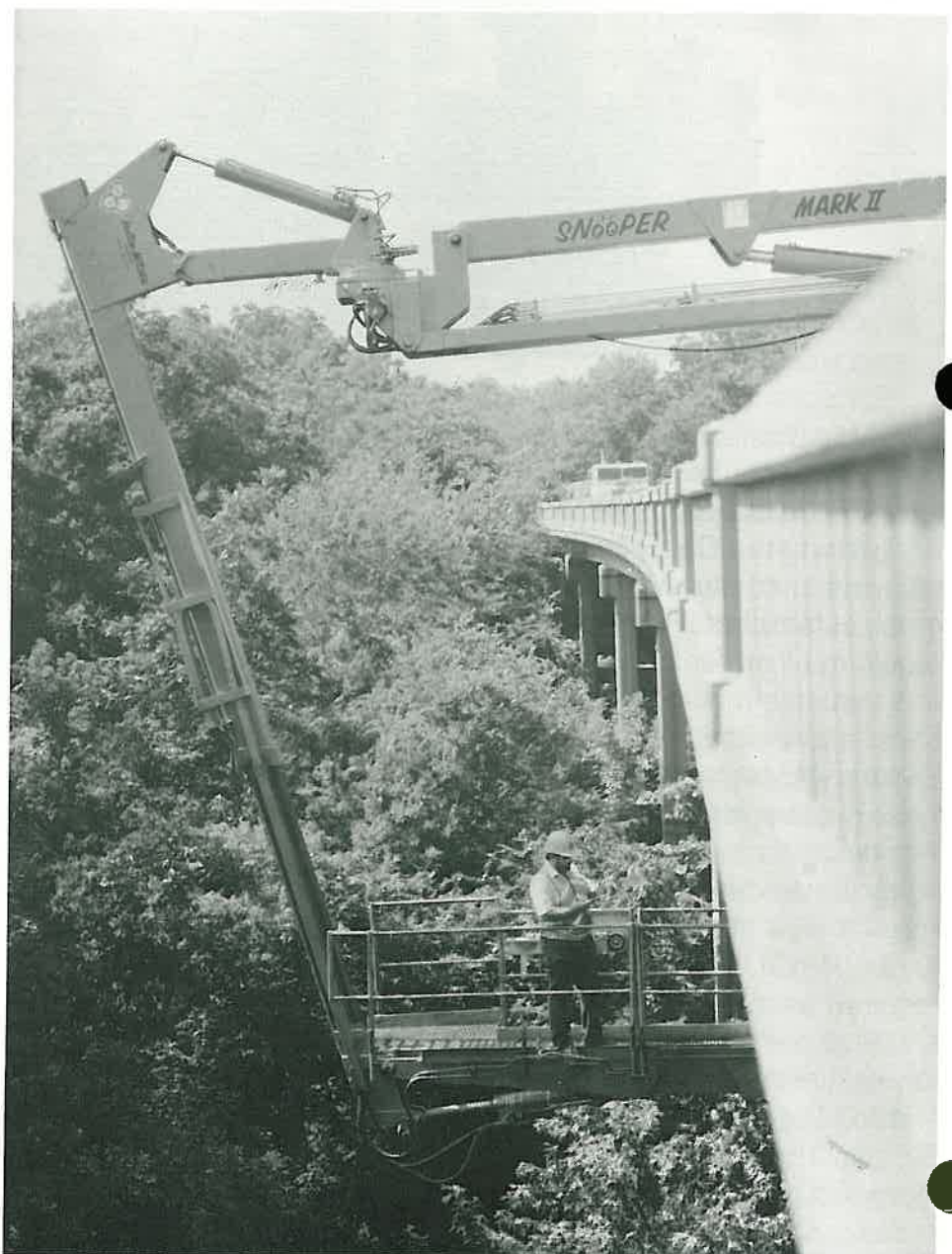
An AHTD Bridge Inspector utilizes the "Snooper" to check underneath a bridge structure.
