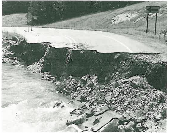
Above photo: Sections of roadways were completely washed out by the May flood.
