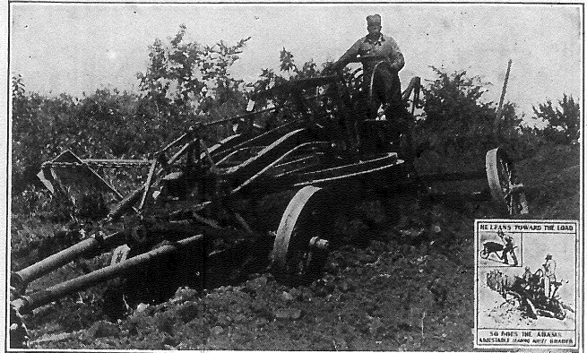
Adams 10-ft. Grader finishing a ditch bank by making a heavy cut with the Back Sloper. Front wheels leaned to offset side pull of Back Sloper. Rear wheels leaned to hold machine against heavy cut.
