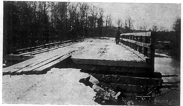
A bridge approach washed out on the Monticello-Tillar road. Practically all bridges suffered like damage.
