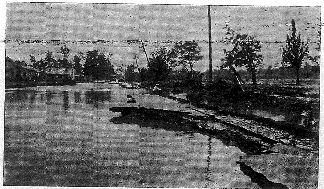
One of the many places where the hard-surfaced road was not only washed out but washed away. This view on Arkansas-Louisiana Highway.
