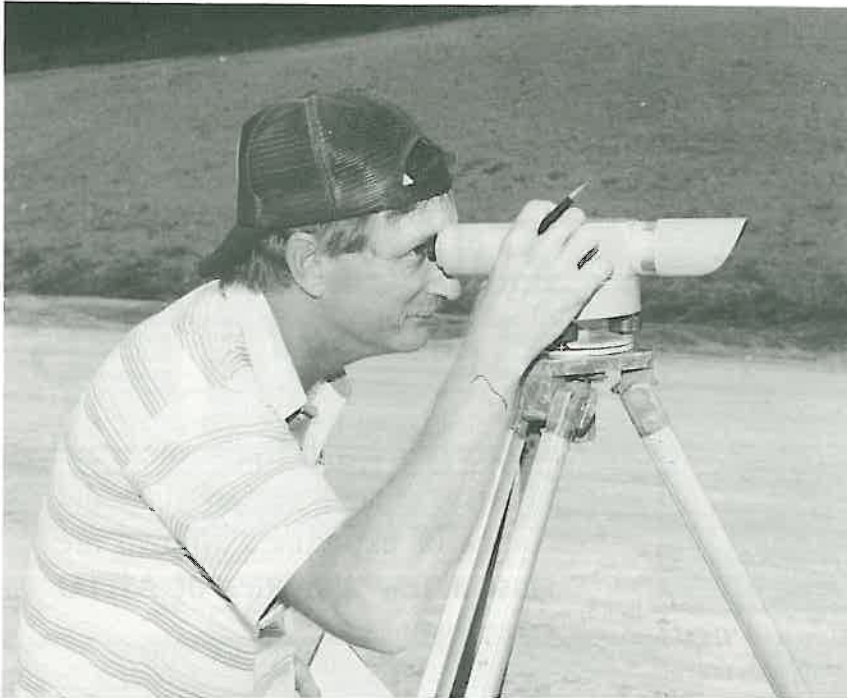
Corky Chamberlain , Construction Aide III for District Six, surveys along a new section of Highway 270 in Hot Springs.
