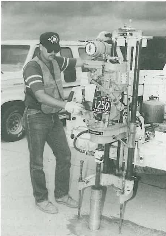
Mark Greenwood , Materials Technician III for the Materials Division, drills for sample cores on the Highway 16 bridge at Heber Springs.
