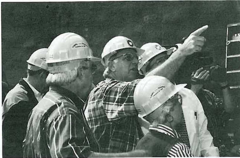
AHTD Director Dan Flowers, center, points to the retaining wall construction around the tunnel portals.
