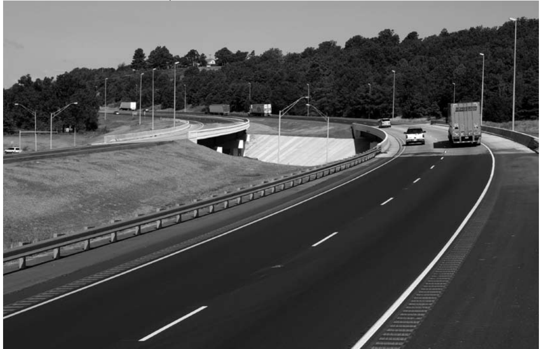
Included in the project were reconstructing the main lanes and two bridges, and updating all safety devices.
