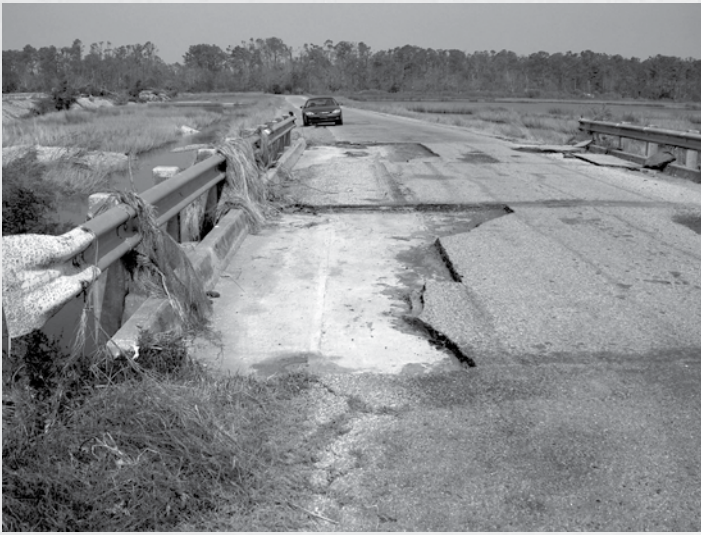
A Waveland, Mississippi, bridge sustained substantial damage on the deck surface.
