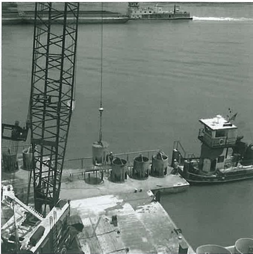
Buckets of concrete are lifted onto the bridge structure from a barge on the river.
