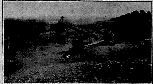
No. 12-B Pioneer Screening, Crushing and Loading Plant and Pioneer Power Unit in operation at Walsenburg, Colorado. This Plant is the property of Mountain States Construction Company, Pueblo, Colorado.
