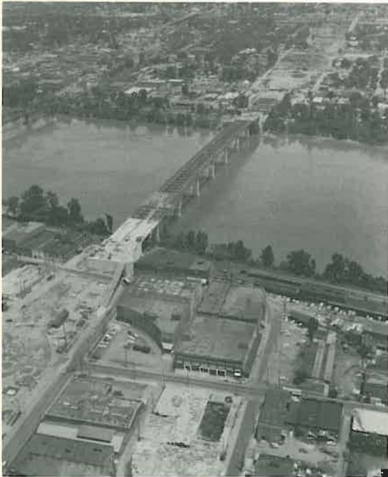
The concrete deck on the Freeway Bridge is partially complete, as this aerial view shows. The view is looking towards North Little Rock.
