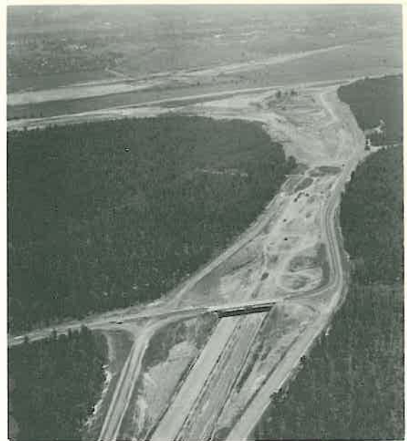
This view on Highway 67, is looking toward the Dark Hollow Interchange on the Jacksonville pavement. Job No. 6615.
