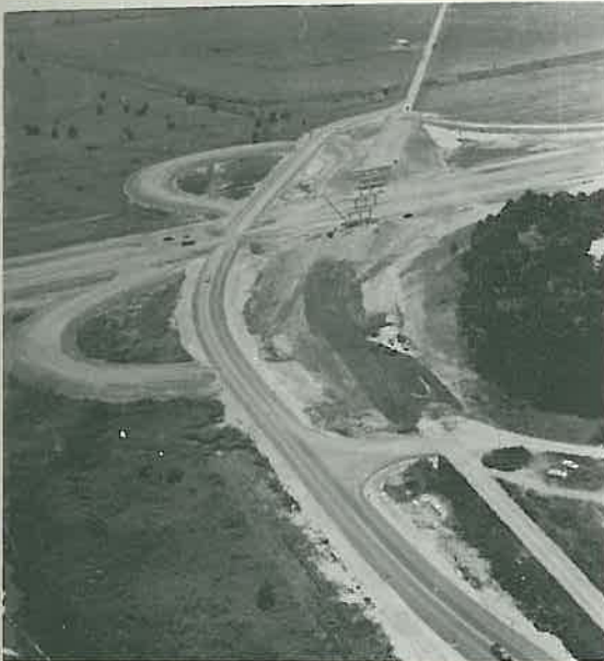
Job No. 6628, Dark Hollow Interchange and Connections, shows the detour and structure carrying 67 W traffic over Interstate 40.
