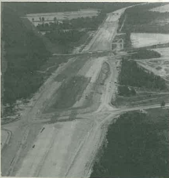
Job No. 6647. Construction at Sixty-fifth Street and RR crossing, looking toward Industrial Spur-Fourch Interchange.
