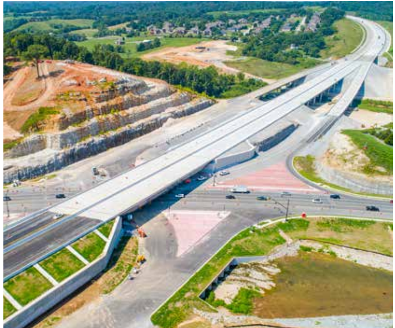
A CAP project at the Highway 71 Interchange on the Bella Vista Bypass
