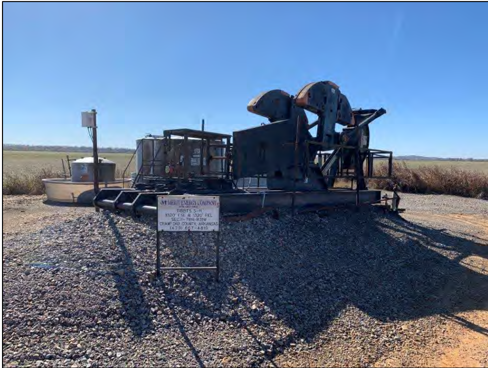
Photo 19: View north of Merit Energy Company, LLC. – Tibbitts #5-11 well head ( Exhibit 2, Map ID #8 ) located west of Thornhill Street south of Kibler. Well head on right side of pump jack.
