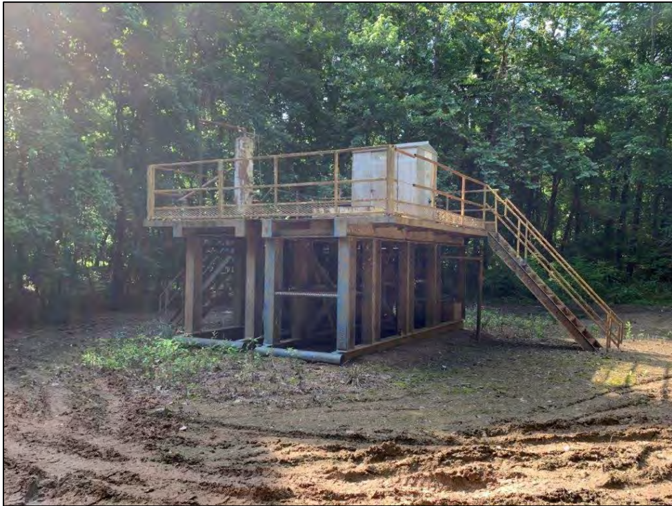
Photo 27: View northeast of skid mounted gas/water separator at Fort Chaffee Federal 1-27 wellhead.
