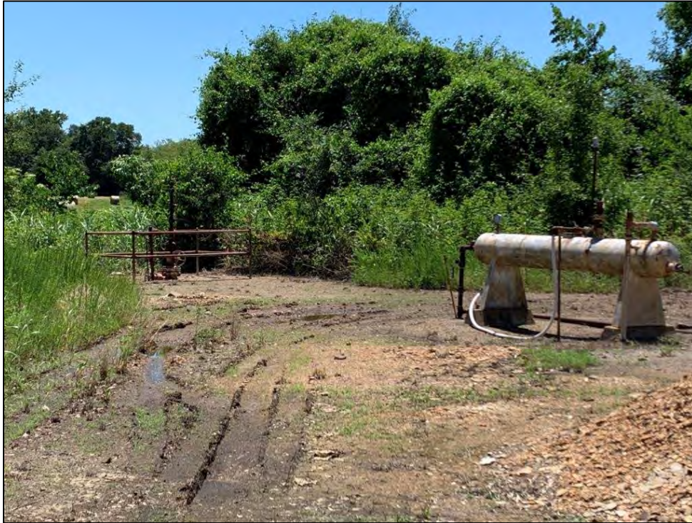
Photo 3: View west/southwest of Brown 1-1 wellhead (Exhibit 2, Map ID #3) with gas/water separator.
