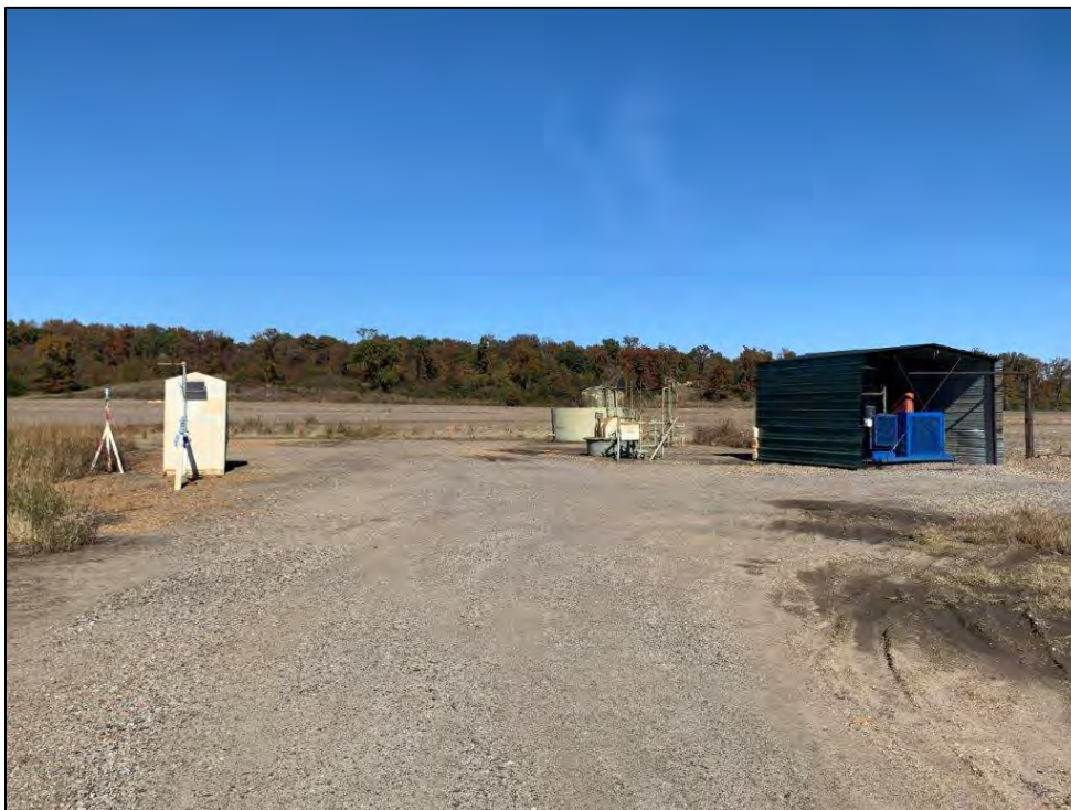
Photo 8: View north of Stephens Production – Newton, Don #1 well head ( Exhibit 2, Map ID #4 ) located east of Thornhill Street south of Kibler. This wellhead had a diesel-powered compressor.
