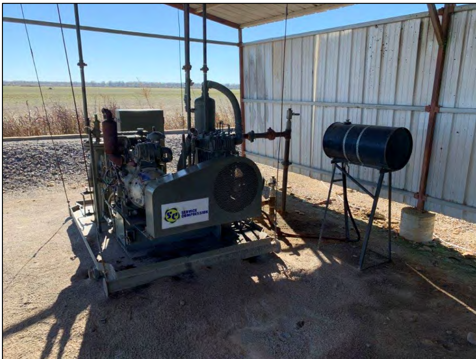
Photo 20: Well head compressor near Tibbitts #5-11 well head ( Exhibit 2, Map ID #8 ). Some stained gravel evident.
