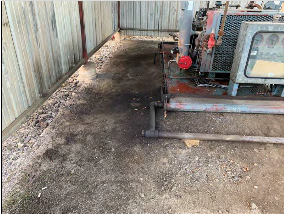
Photo 29: View of oil staining around wellhead compressor at Merit Energy Company, LLC USA 1-34.
