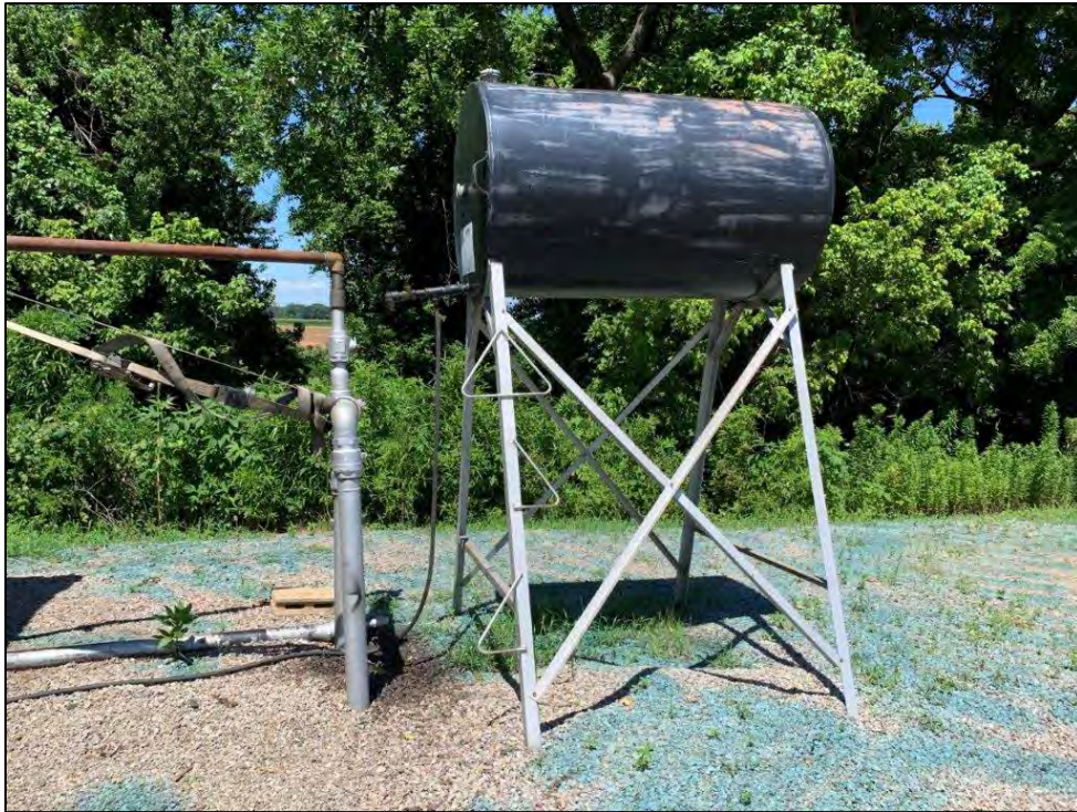
Photo 15: Diesel AST at compressor station near Cazort #8 well ( Exhibit 2 Map ID #19 ). Green herbicide staining also visible.
