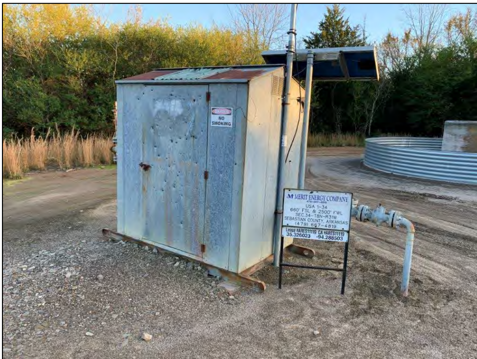
Photo 28: View south of Merit Energy Company, LLC USA 1-34 well head sign. approximately 0.1-mile north of E. Church Street.
