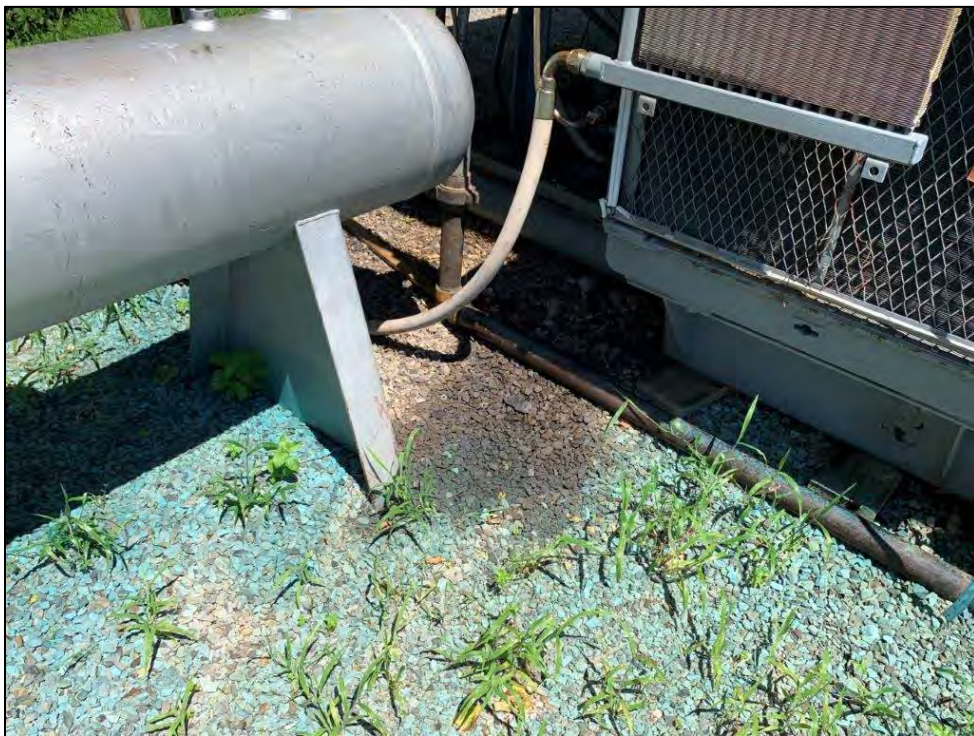
Photo 14: Oil staining below compressor at location above. Green herbicide staining also visible.
