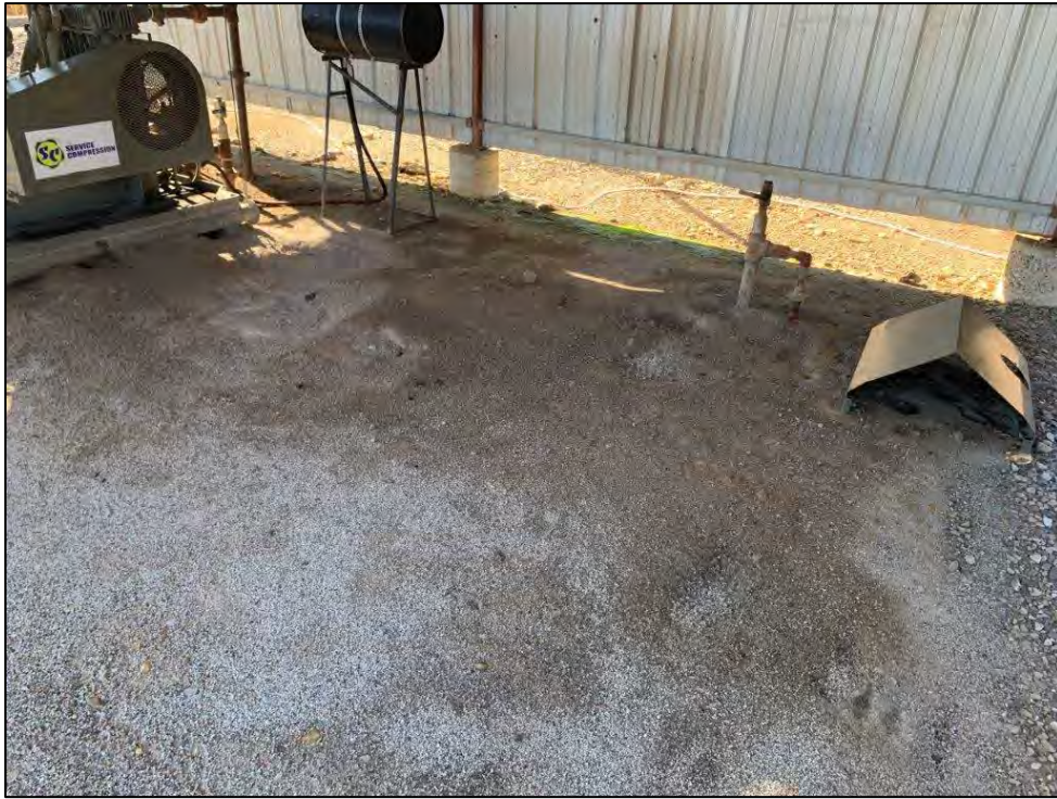
Photo 21: View of stained gravel near compressor at Tibbitts #5-11 well head (Exhibit 2, Map ID #8).
