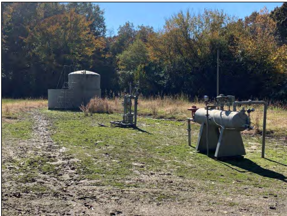
Photo 6: View south of Stephens Production – Newton, Don #2 well head ( Exhibit 2, Map ID #5 ) located east of Thornhill Street south of Kibler.
