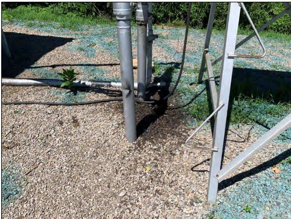
Photo 16: Oil staining below AST at location above. Green herbicide staining also visible.
