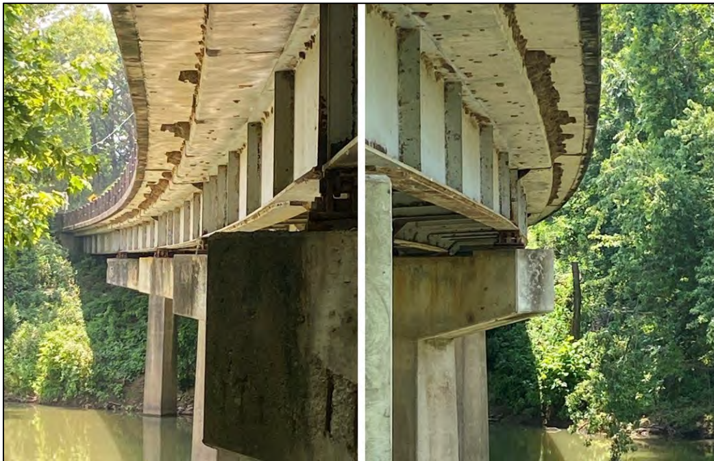
Figure 6-3: Cliff Swallow Nests on the I-49 Ramp off of I-40 over Frog Bayou
