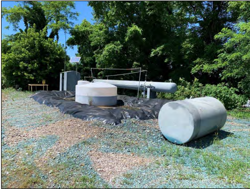
Photo 13: View northwest of produced water tank and gas-water separator ( Exhibit 2 Map ID #19 ) near Cazort #5 and #8 wells. Green herbicide staining also visible.
