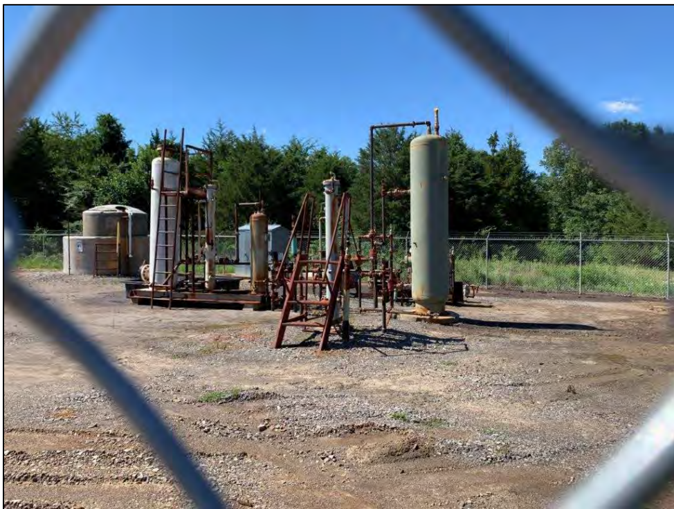
Photo 24: View northwest of gas/water separators and produced water tank.
