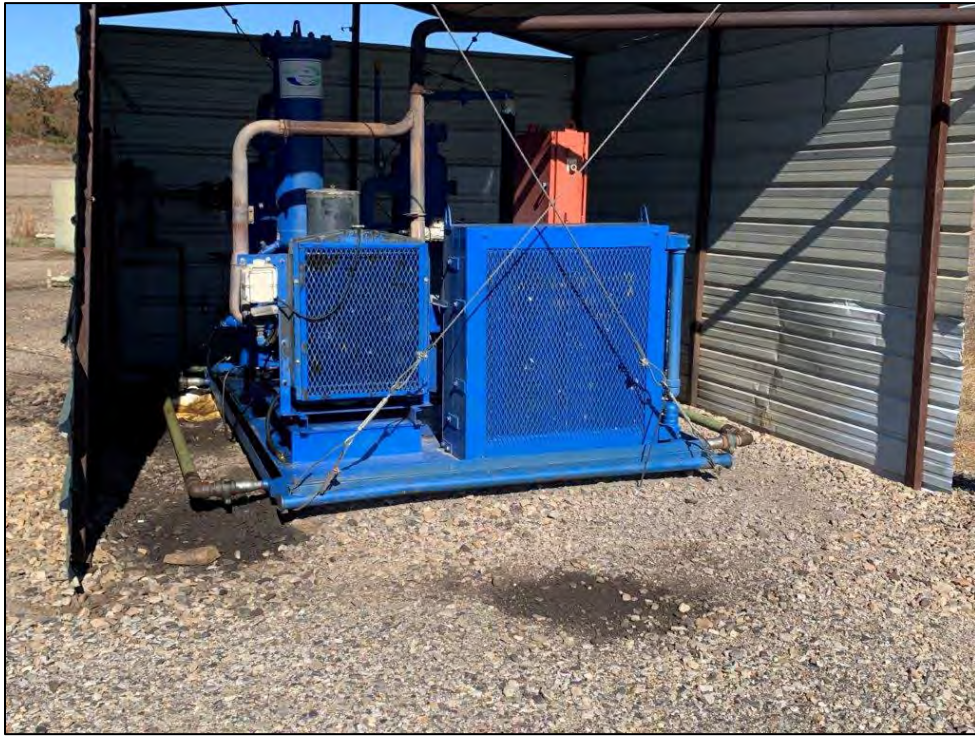
Photo 9: Oil staining on gravel around diesel-powered compressor at Stephens Production – Newton, Don #1 well head.
