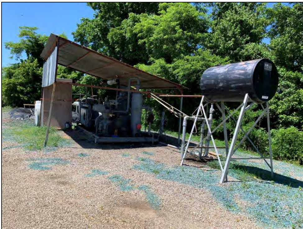
Photo 12: View northwest of compressor ( Exhibit 2 Map ID #19 ) and diesel AST located southeast of Cazort #8 well. Green staining is liquid herbicide sprayed for presumed weed control.
